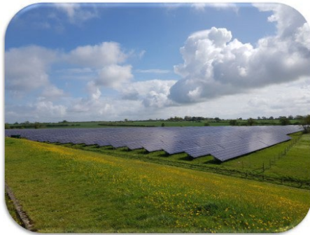
Solar farm at Grafham Water
